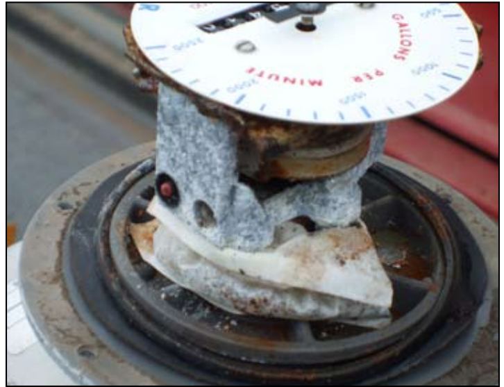
This pictures shows what can happen to a register without a canopy boot. Regular inspection and maintenance could have prevented costly repairs or replacement with this meter.
